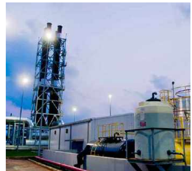
UthuruJanani Power Plant / Itl.lk
